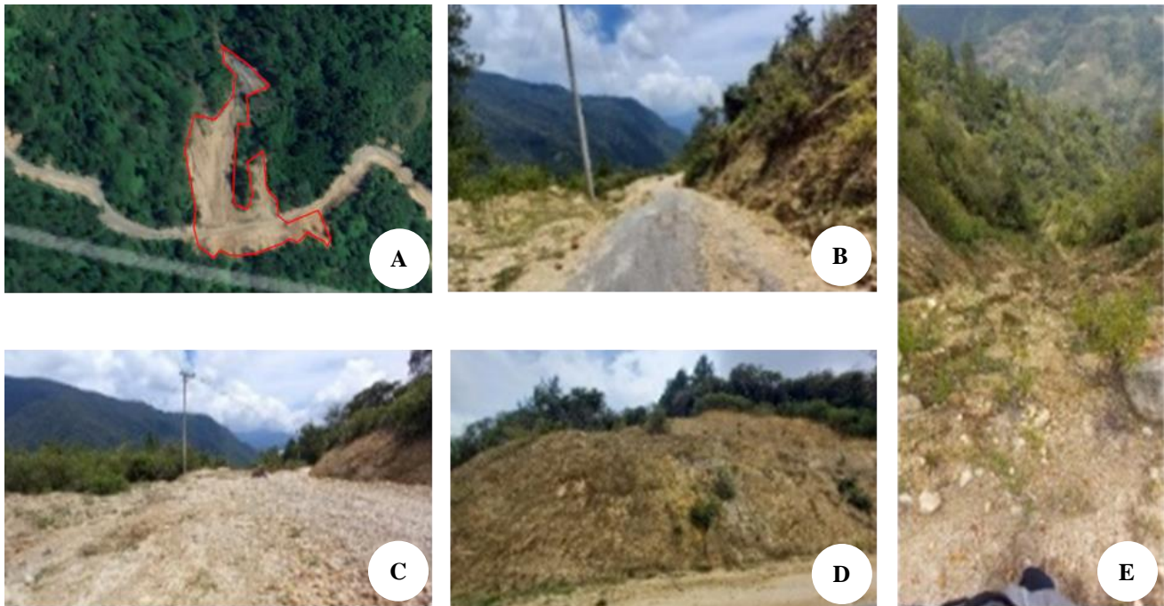
Figure 2. Landslides in the Rongkong Watershed. A. Interpretation results from Google Earth Pro; B-E. Ground check results
